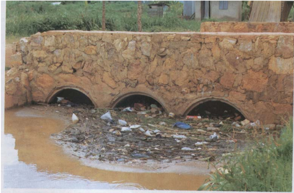
Plate 6.3: Solid waste disposal in drainage channels
